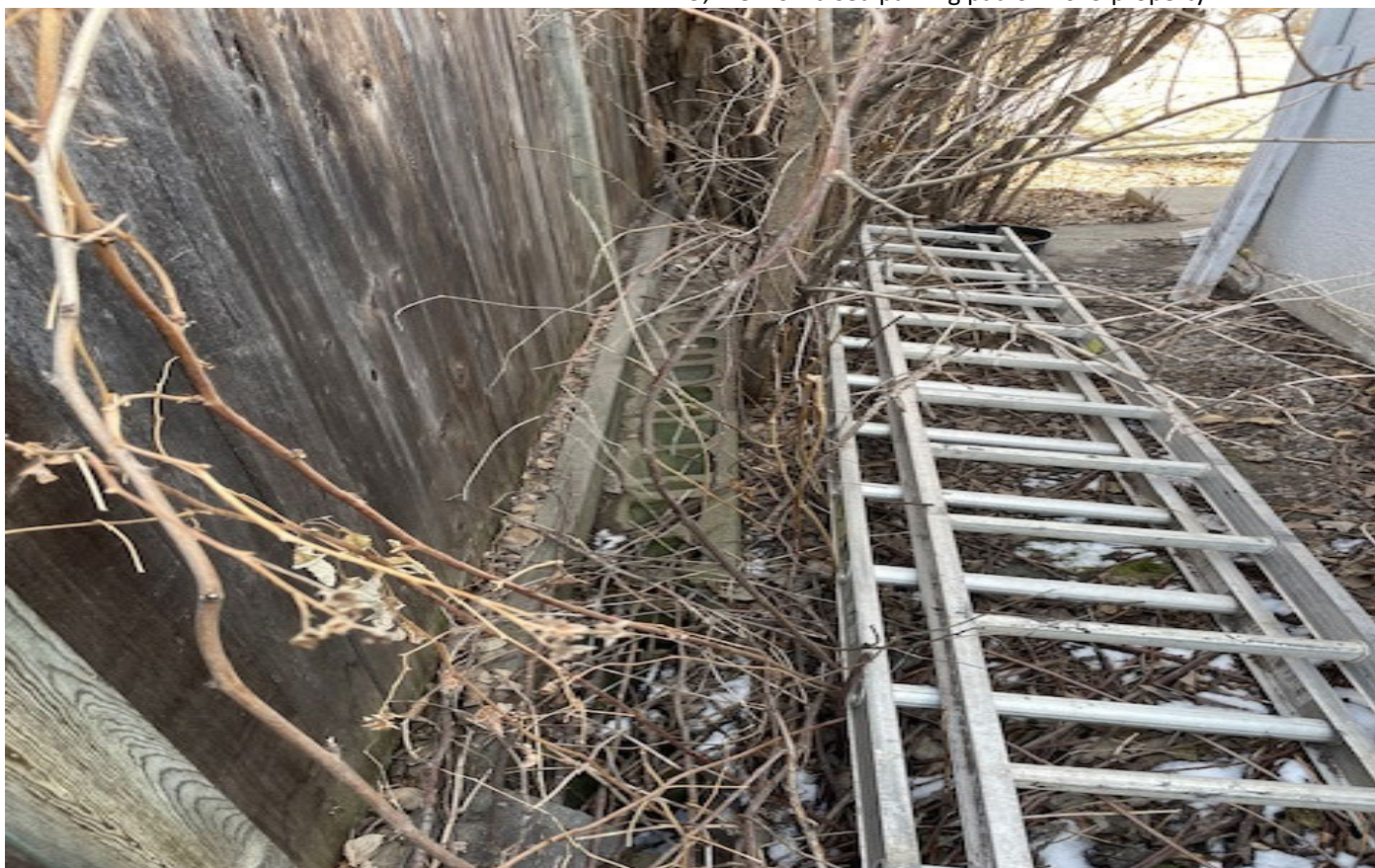
10, View from back alley looking Eastward on 1619 property showing existing concrete block retaining wall.
